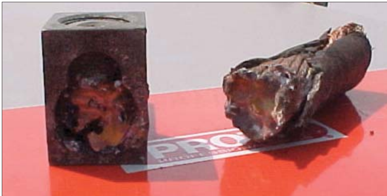
Photo 3. Failed terminal and cable
