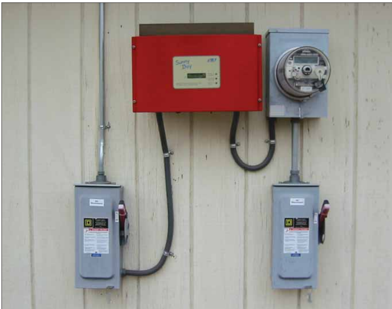
Photo 5. Inverter ac disconnect combined with the utility disconnect to the right of the inverter
