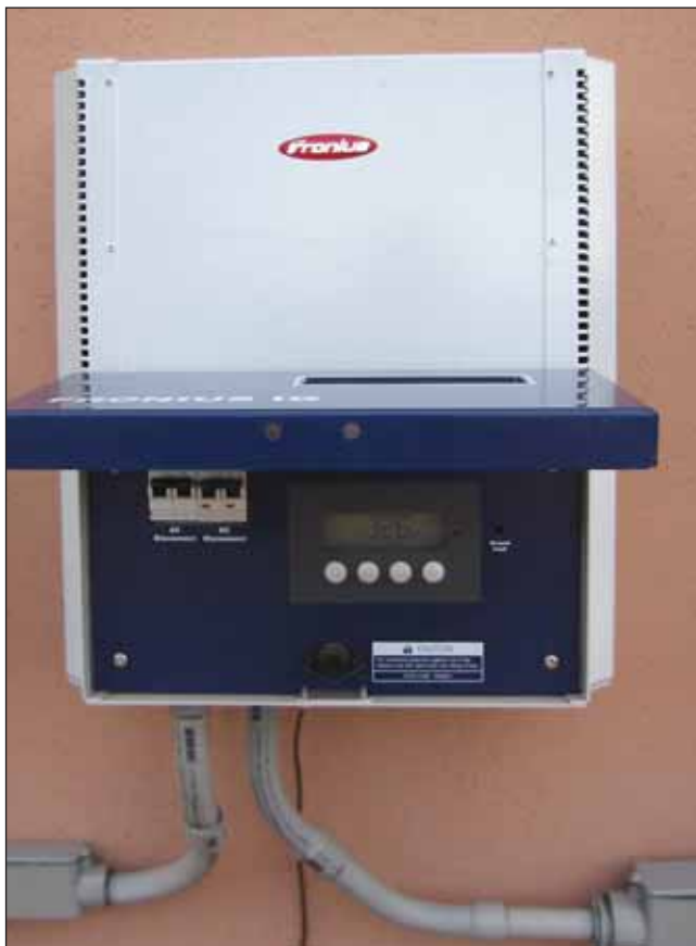
Photo 3. Inverter with internal ac and dc disconnects
