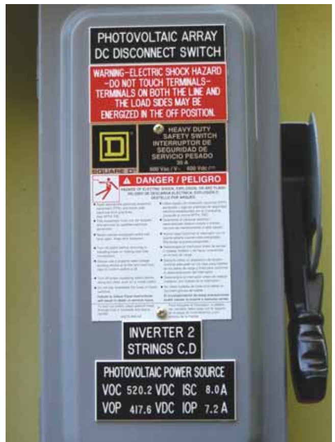
Photo 2. DC PV disconnect with required markings
