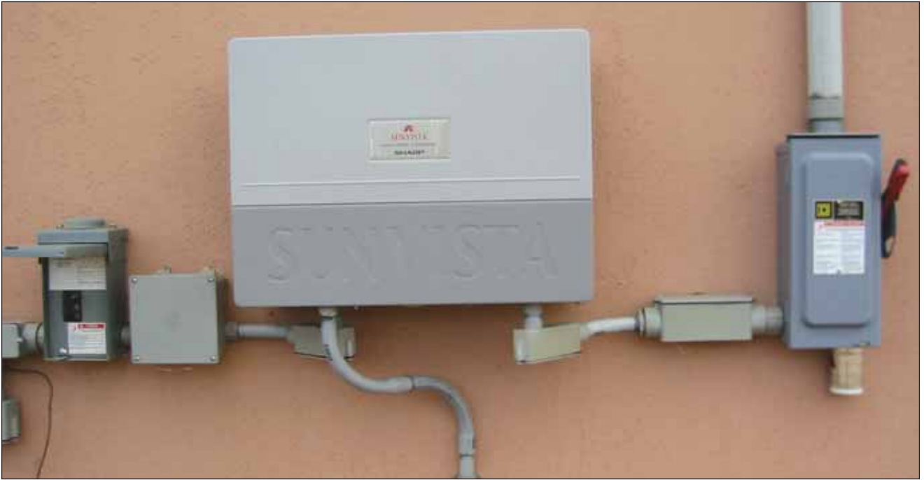
Photo 4. Inverter with external ac and dc disconnects
