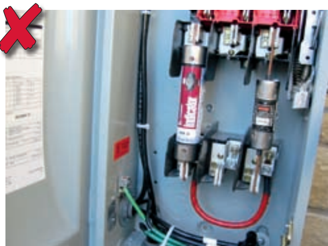
Improper enclosure grounding: wrong device, wrong location.
