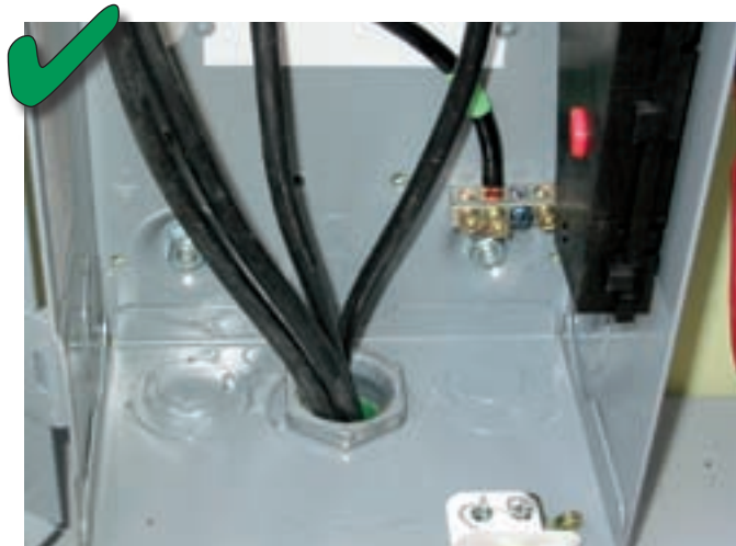
A listed ground-bar kit in the proper location.
