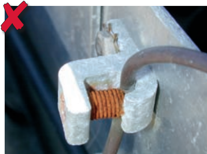
A dry-location lug used in a wet location.
