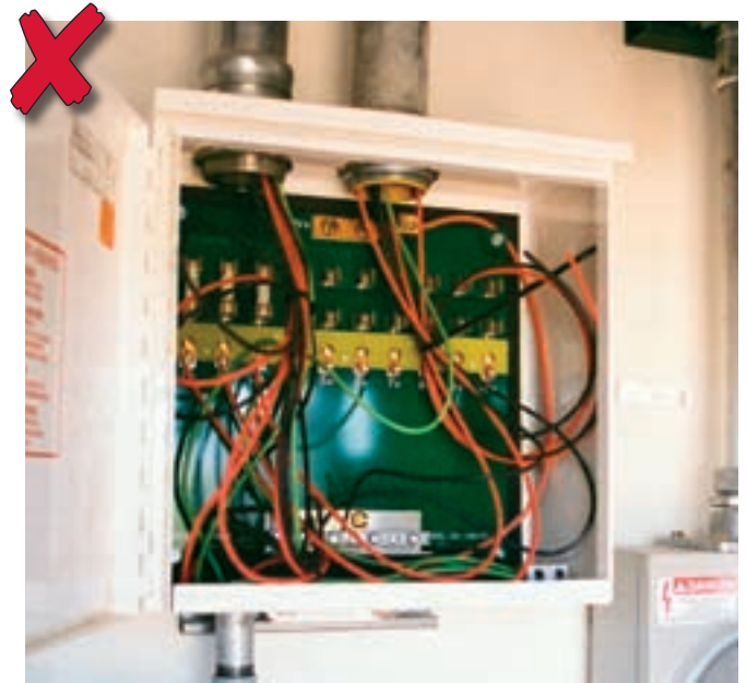
Grounded PV source circuits, but no white conductors.
