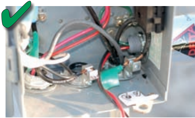
Bonding bushings on 500 VDC conduits.
