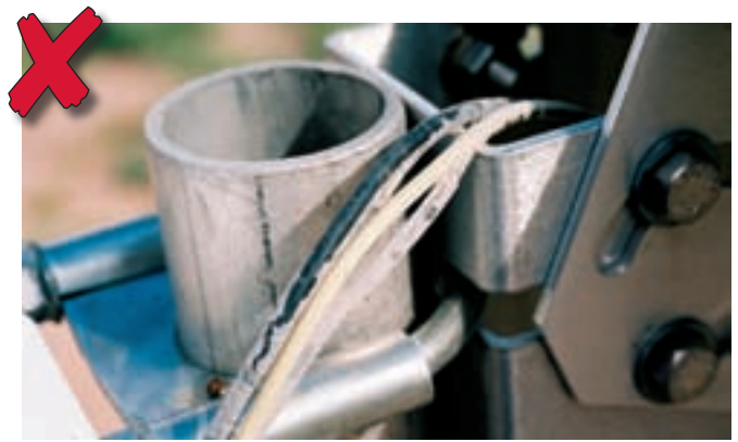
Deterioration of THHN conductors due to outdoor UV exposure.
