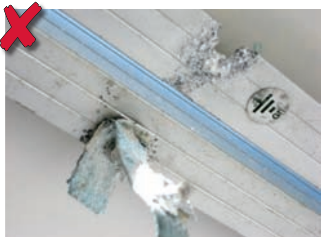
Improper module grounding with dissimilar metals.
