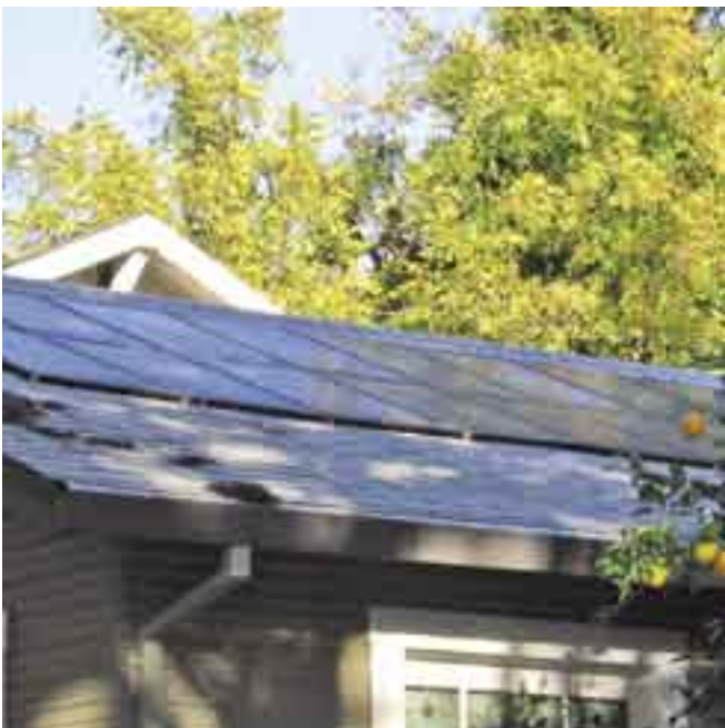
An example of too much shading on a PV array.
