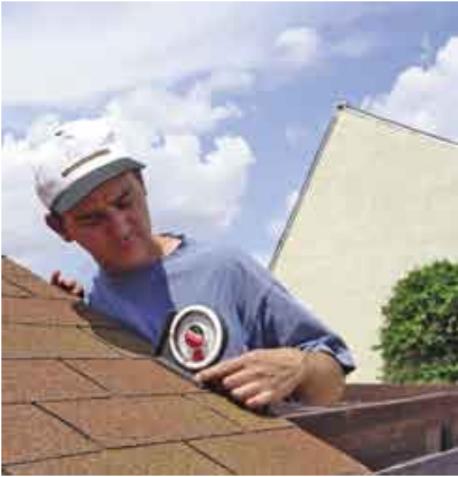
Measure the angle of the roof before installing the array and mounts.
