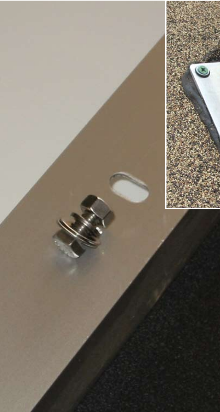
Photo 1. PV module mounting hole and hardware
