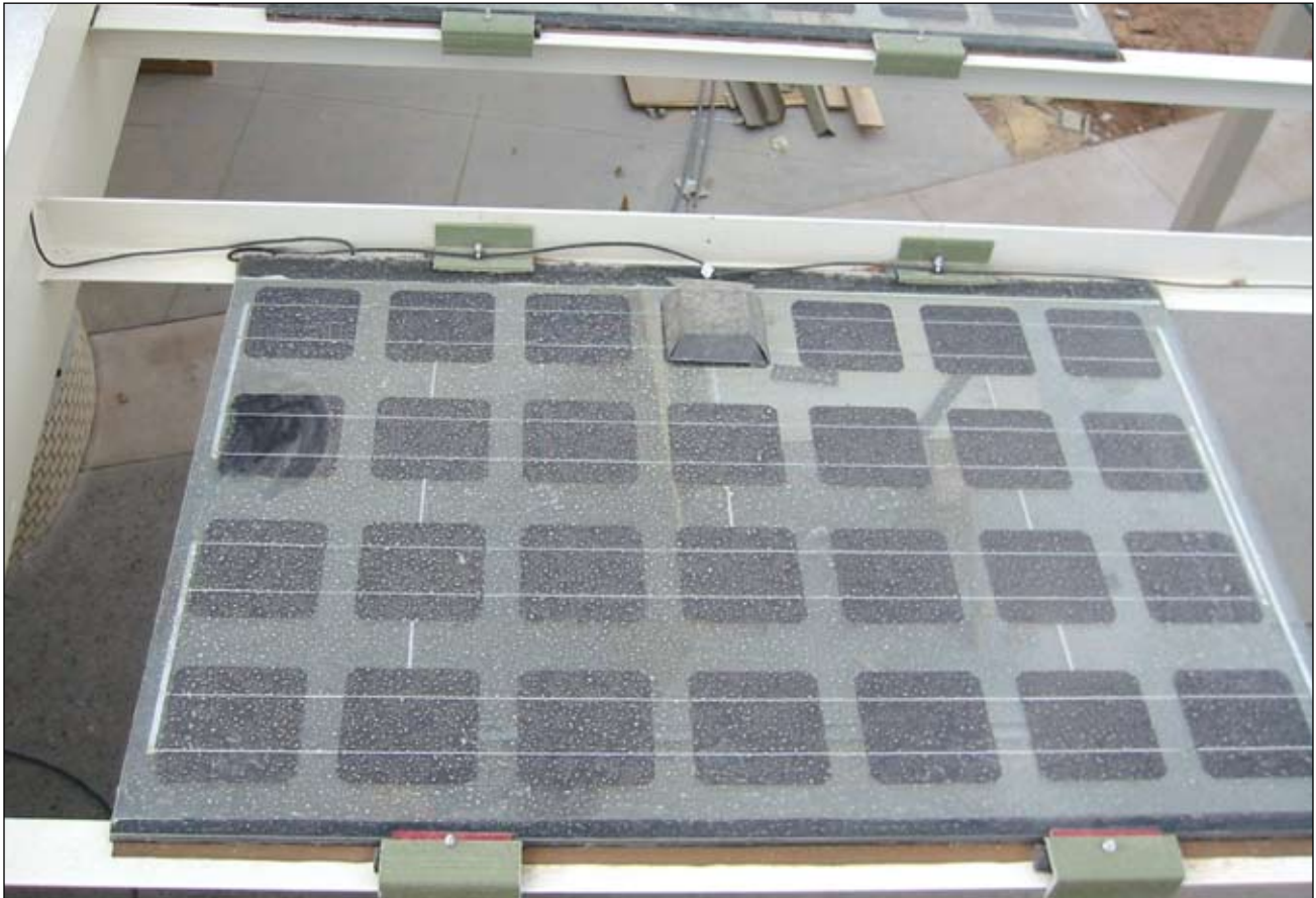
Photo 3. Frameless PV modules in overhead canopy
