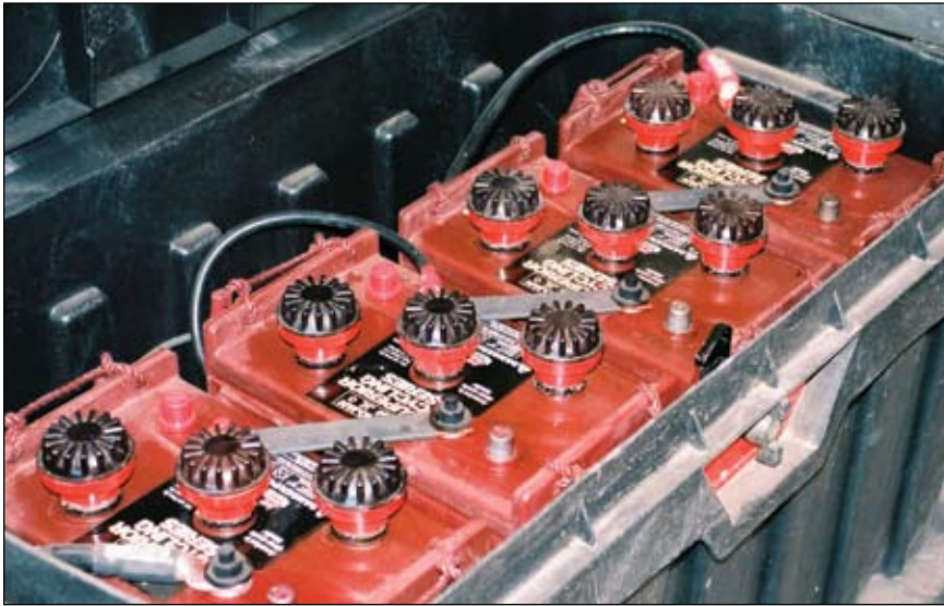
Photo 7. Flooded, lead-acid batteries in containers
