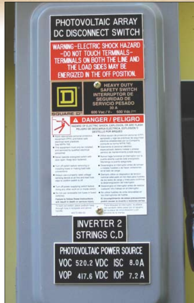
Photo 1. Small system dc PV disconnect
