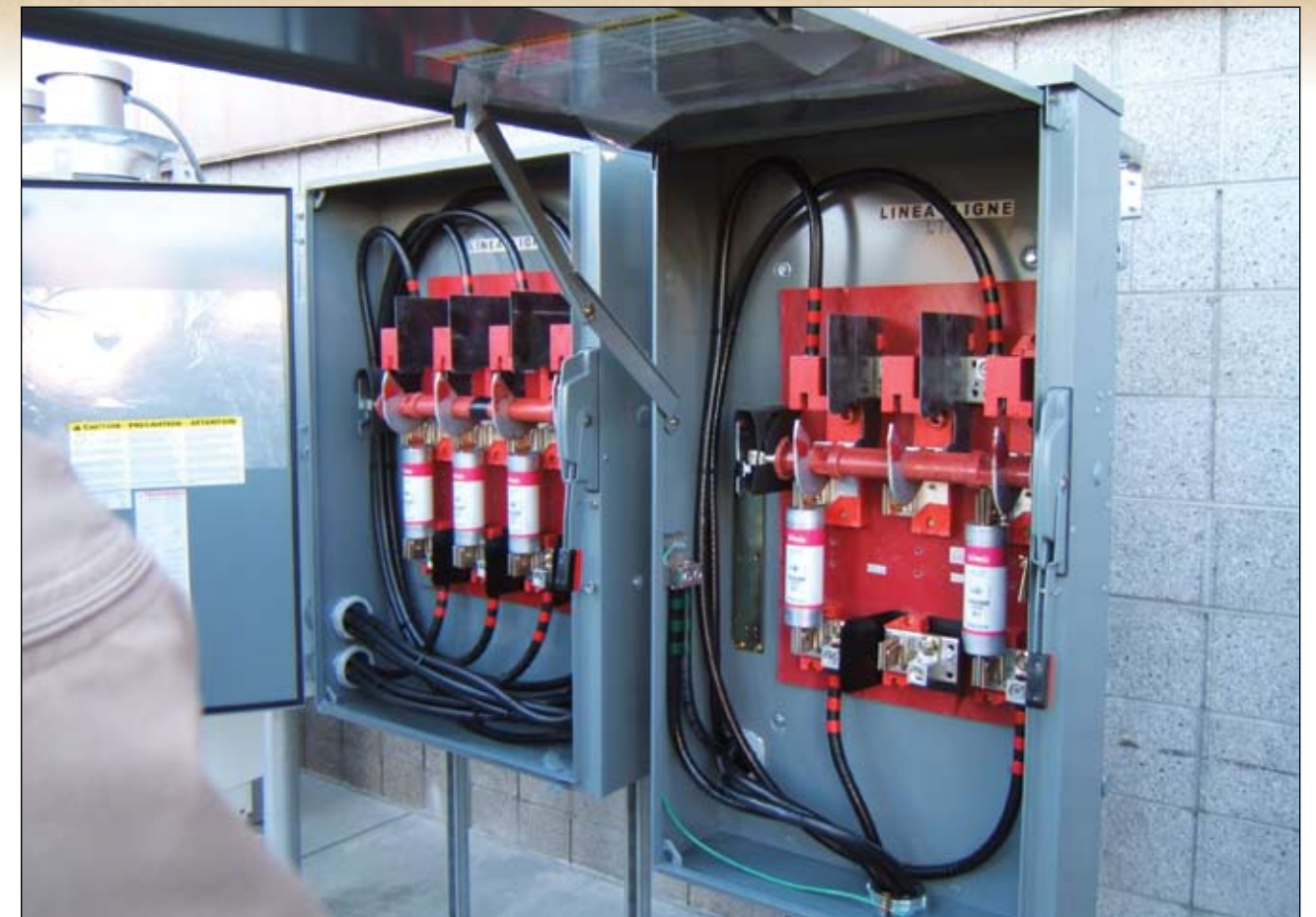
Photo 2. Large system dc PV disconnects
