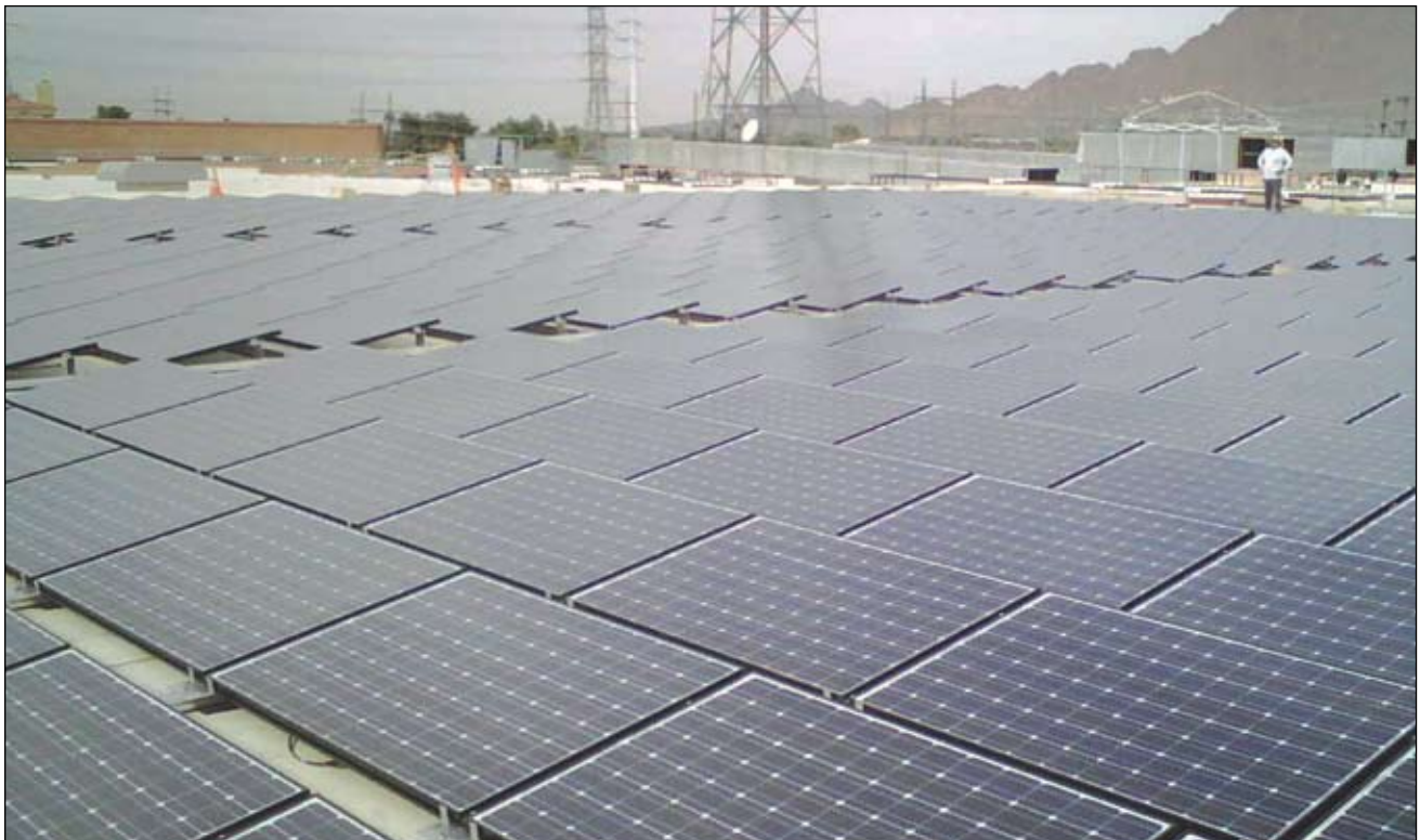
Photo 1a. Large system with multiple strings of modules will require OCPD.
