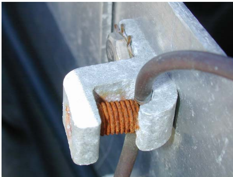
An example of improper component selection and subsequent galvanic corrosion during nine months of outdoor service.
