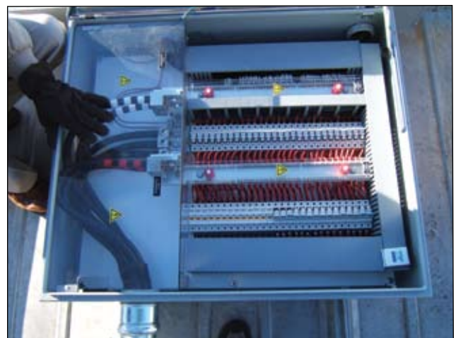
Photo 3. DC combiner boxes with fuses operating up to 600 volts.
