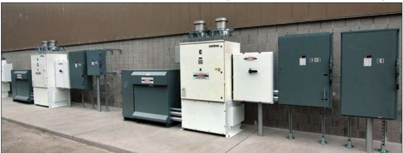
Photo 5. High voltage, high currents—exercise caution!
