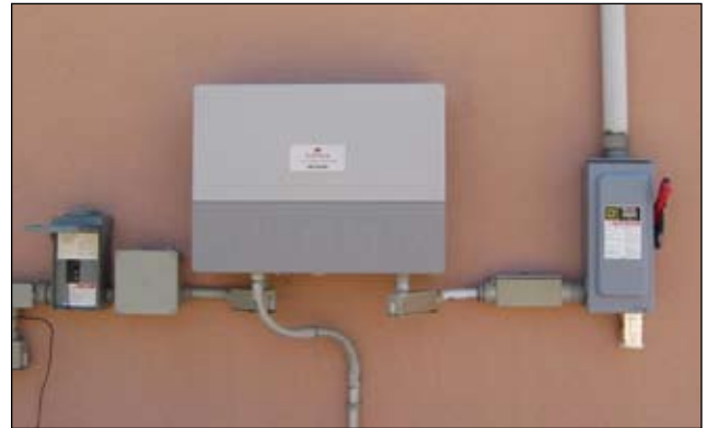
Photo 2. AC and dc disconnects grouped at the inverter
