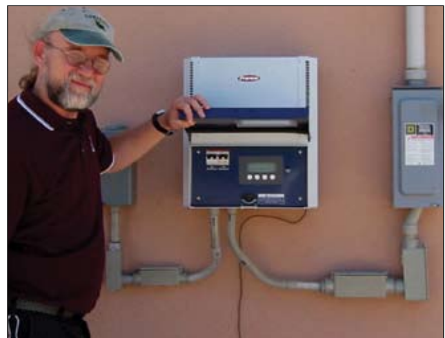
Photo 4. Internal and external dc disconnects
