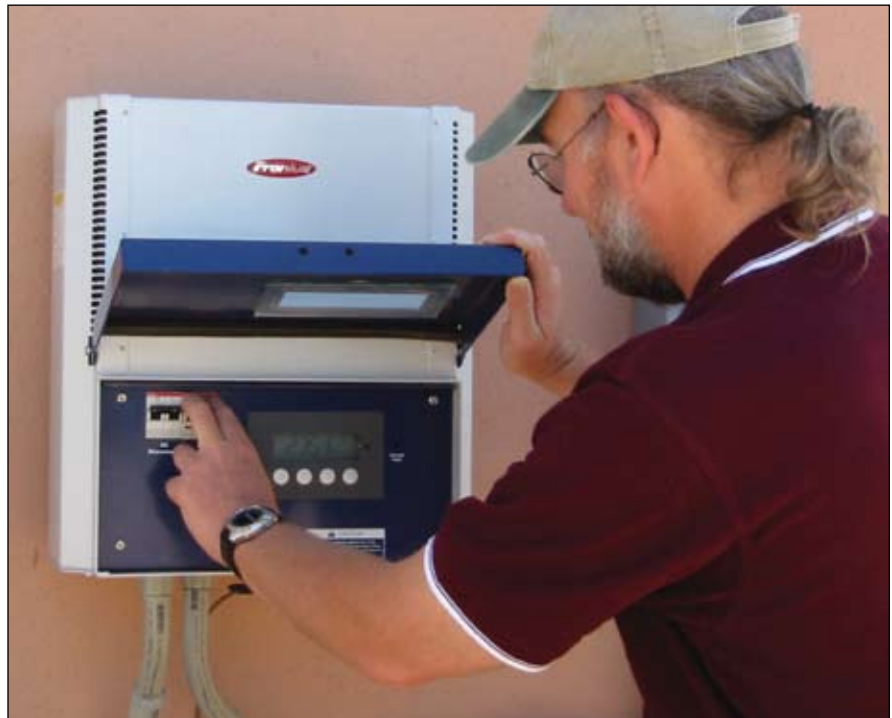
Photo 3. Internal ac and dc disconnects
