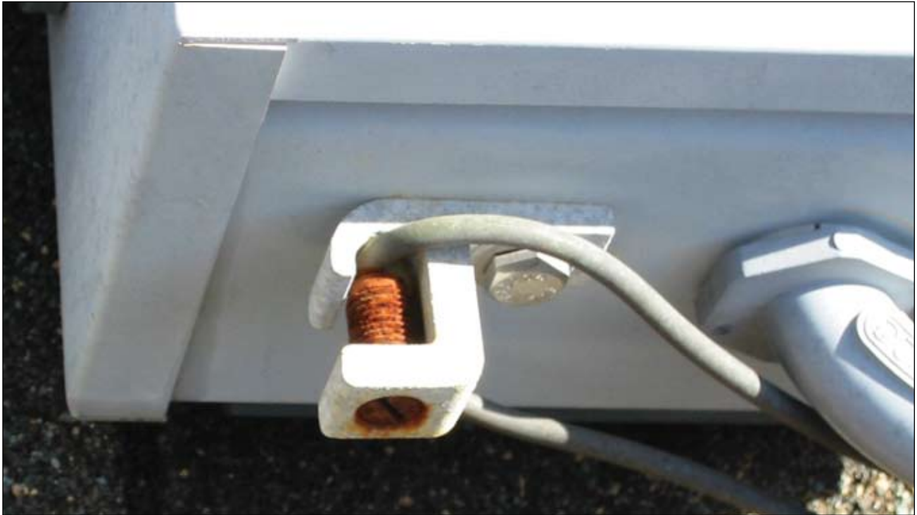
Photo 5. Dry-location lug rusting outdoors
