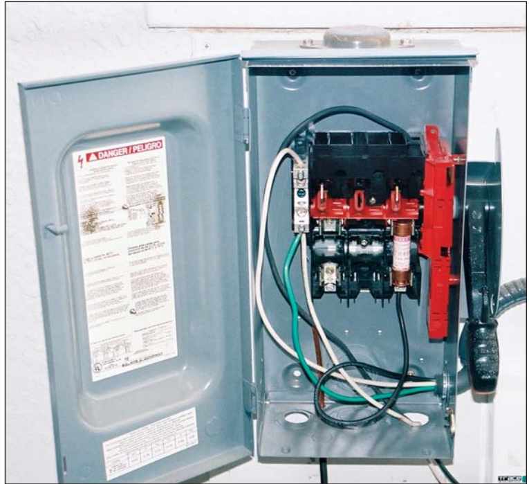
Photo 1. How many conductors can fit in a single terminal?
