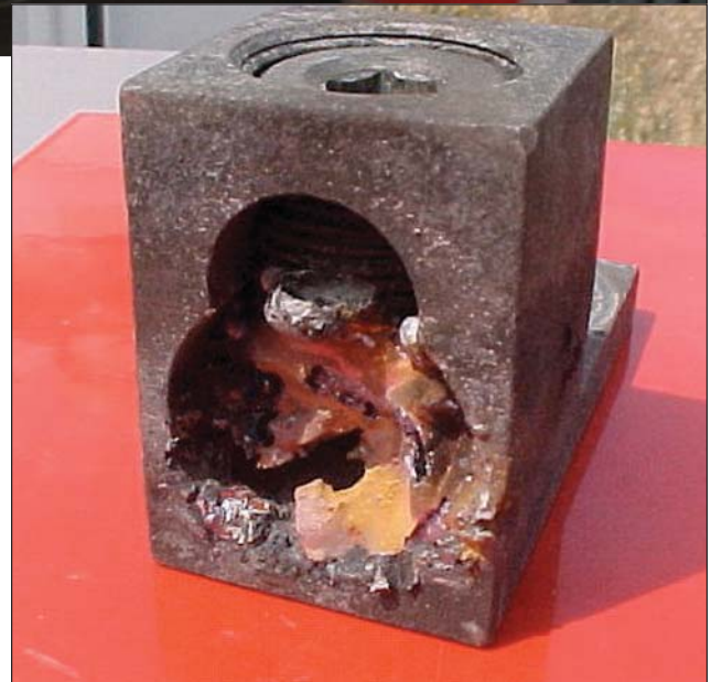
Photo 5. Fine stranded cable, improperly terminated
