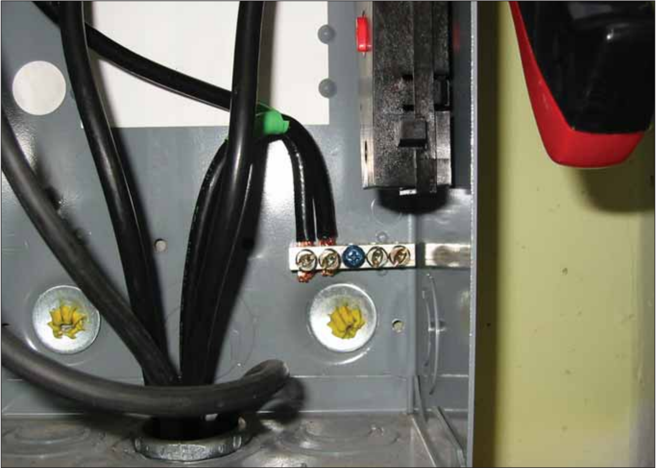
Photo 4. Properly installed, listed ground bar kit
