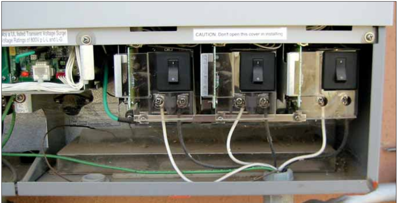
Photo 2. Inverter with three DC inputs
