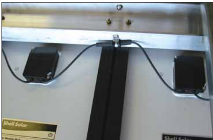
Photo 5. Module wiring properly secured
