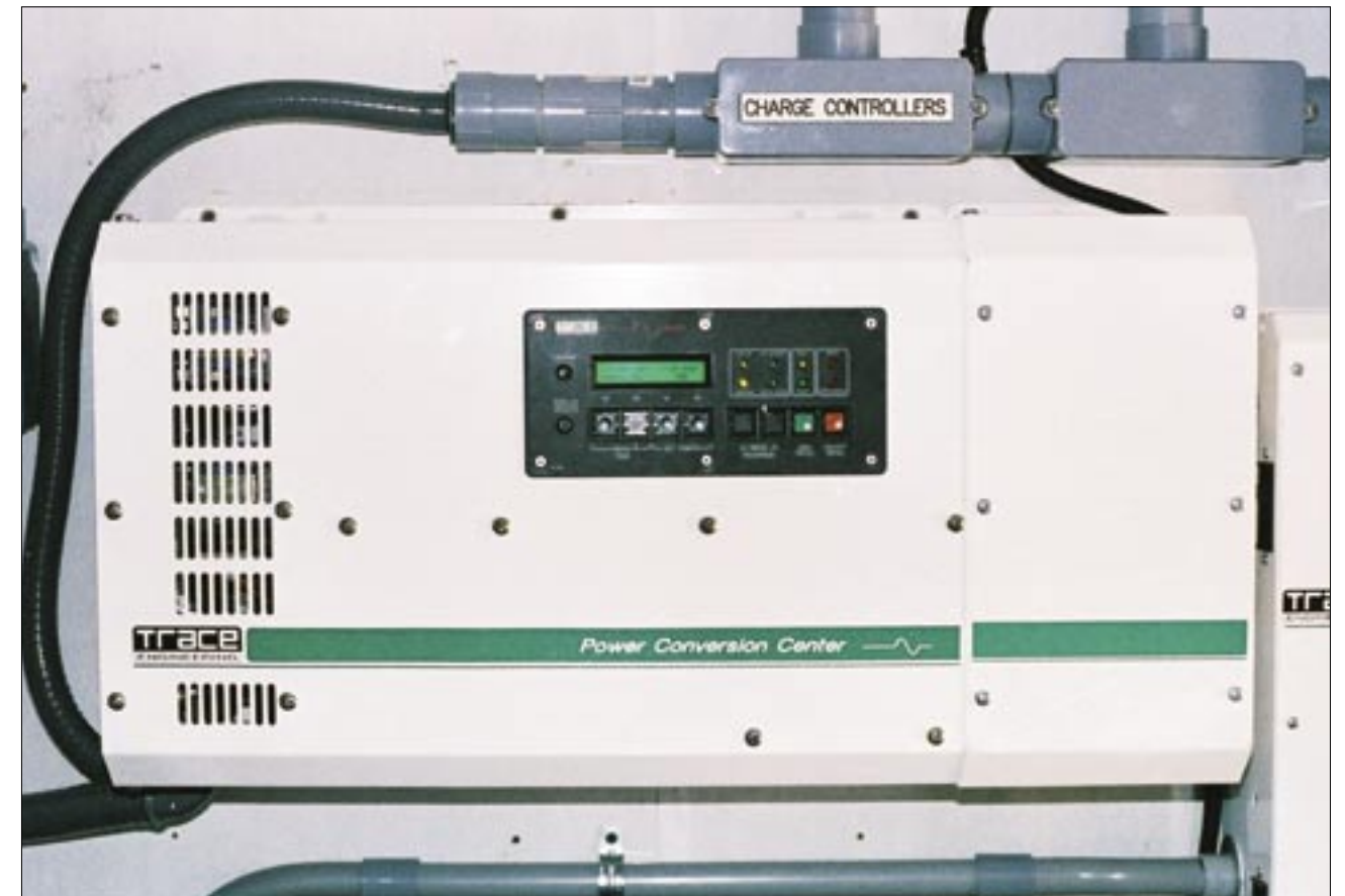
Photo 9. 4 kW stand-alone inverter
