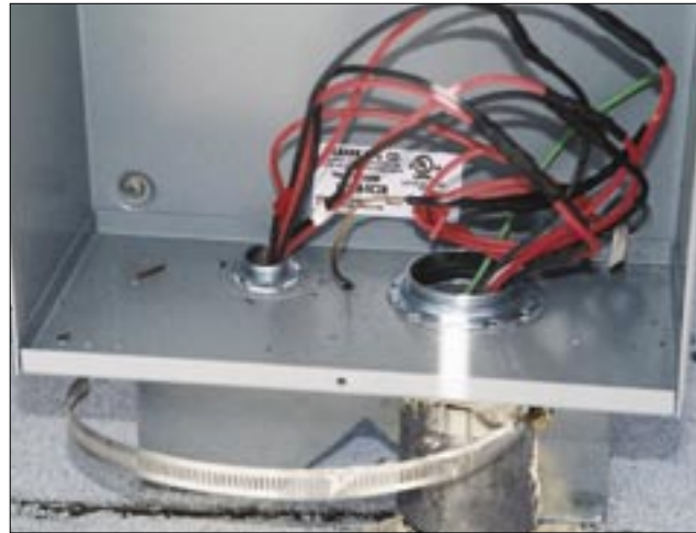
Photo 10. Grounded conductors should be white, not black!
