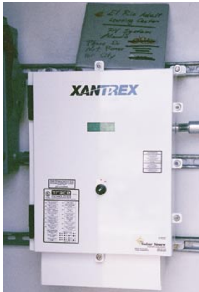
Photo 8. 15 kW 3-phase utility-interactive inverter
