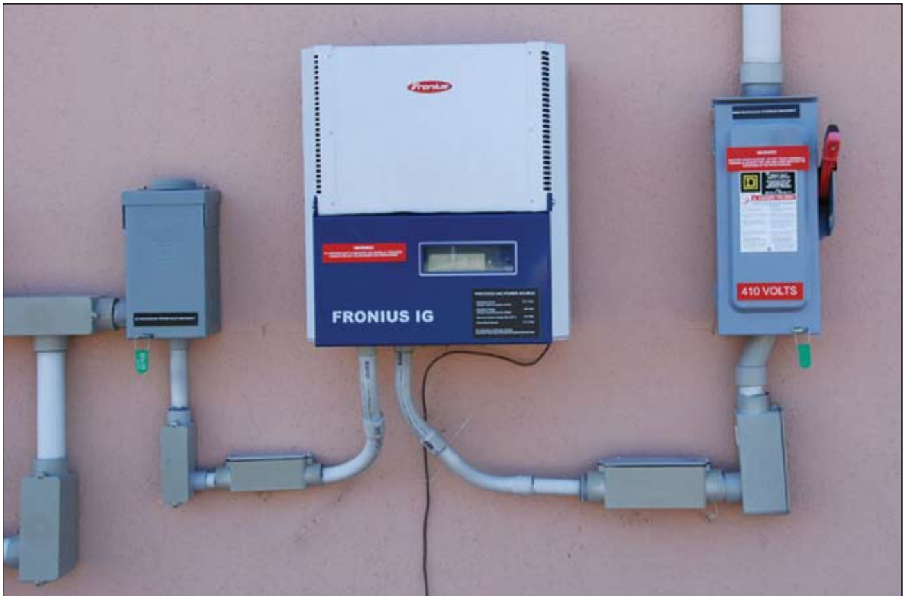
Photo 2. Are they properly grounded?
