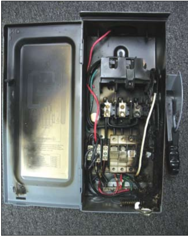
Photo 1. Burned combiner box caused by wiring error
