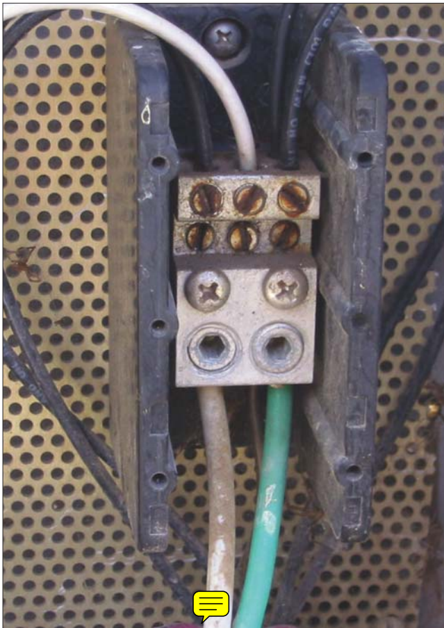
Photo 6. Rust due to improper use of components
