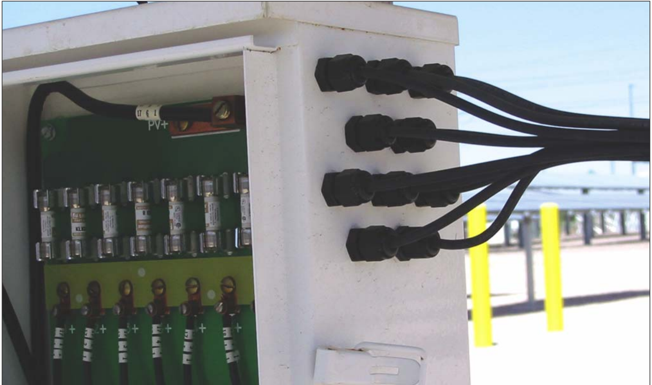
Photo 5. PV combiner in shade
