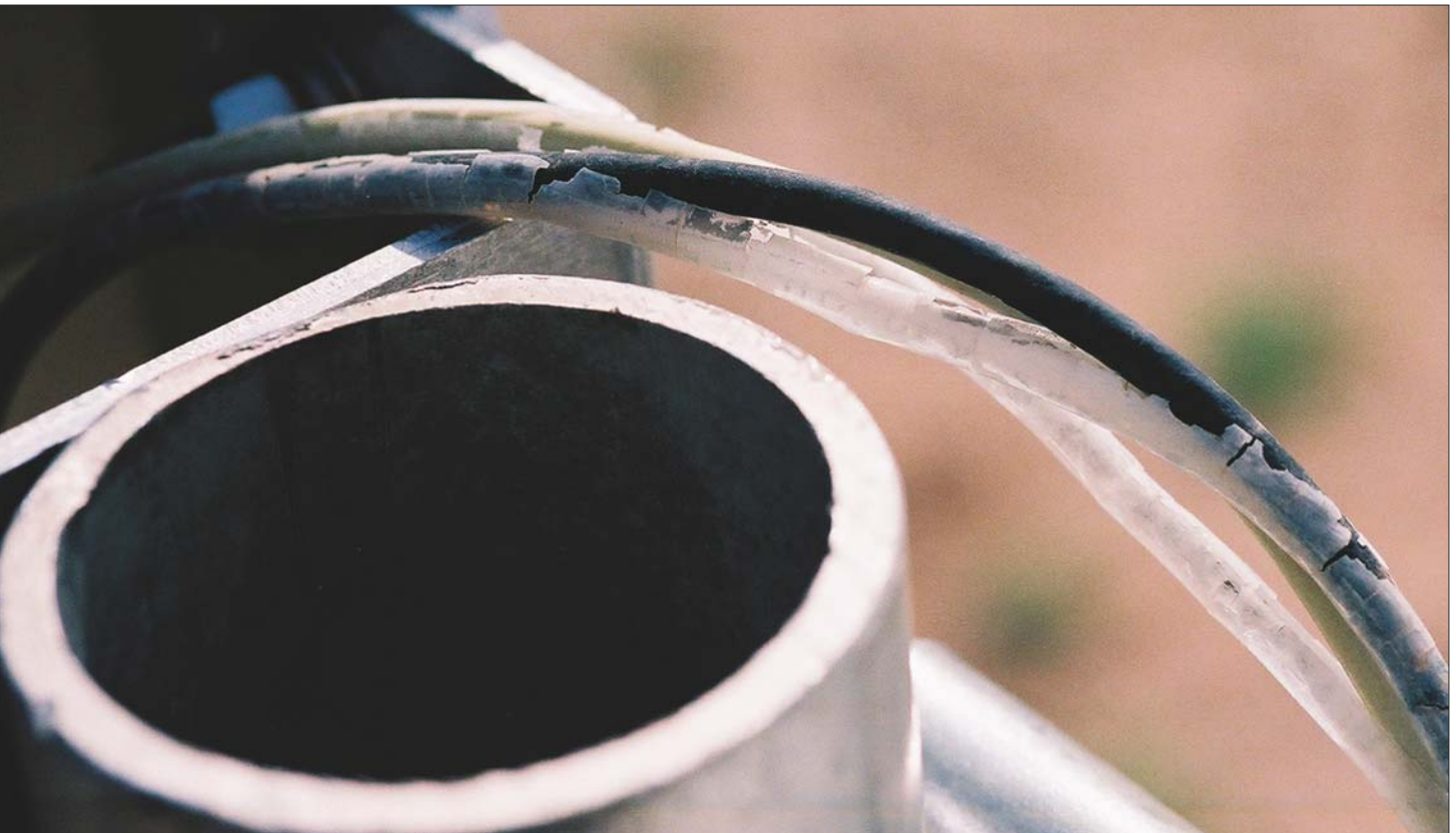
Photo 1. THHN conductors exposed to sunlight
