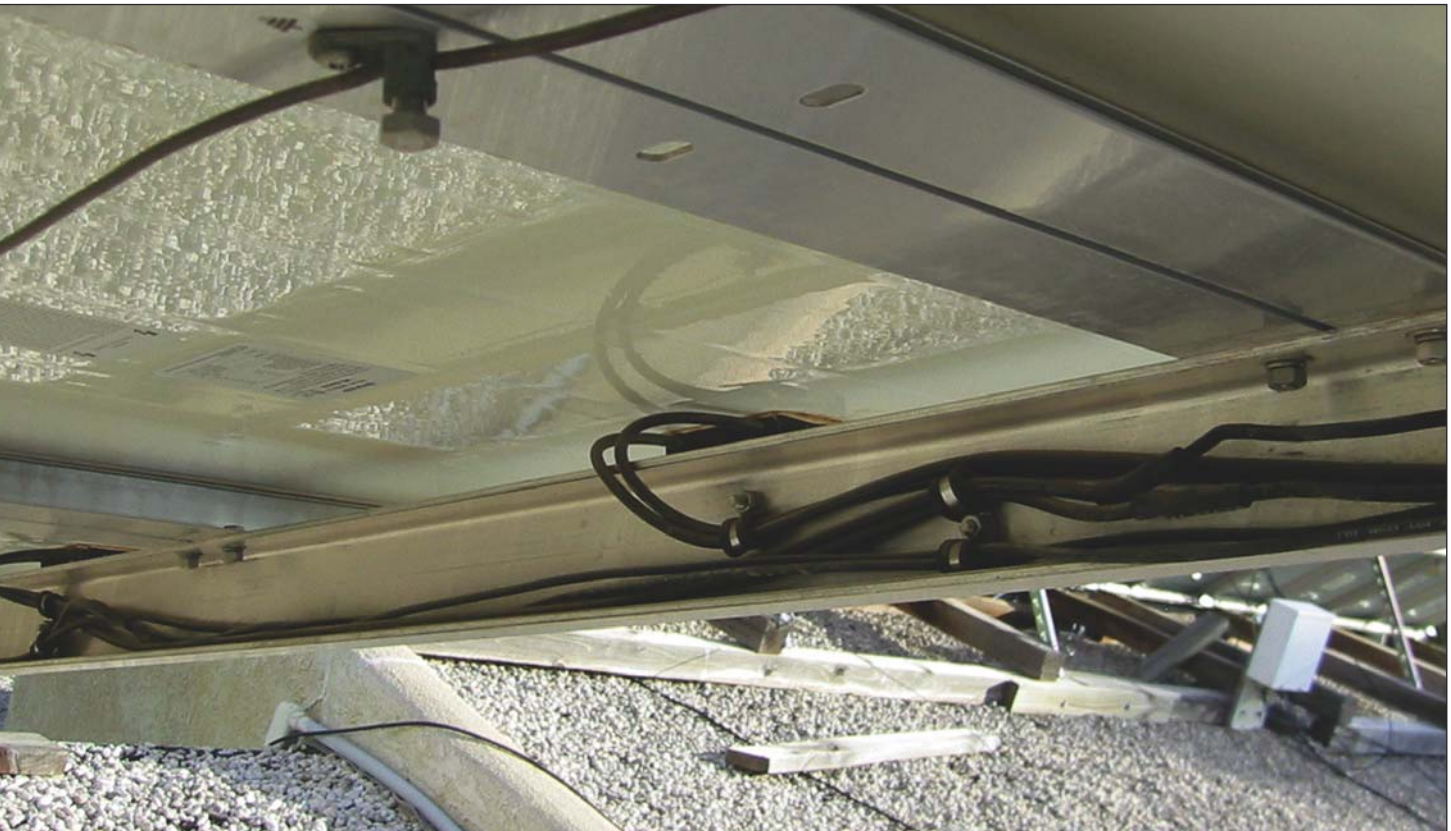
Photo 2. Pipe clamps with inserts holding cables securely
