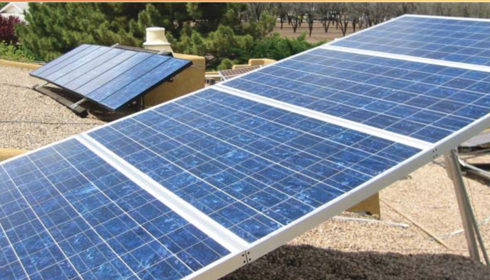
Photo 1. Framed PV modules
