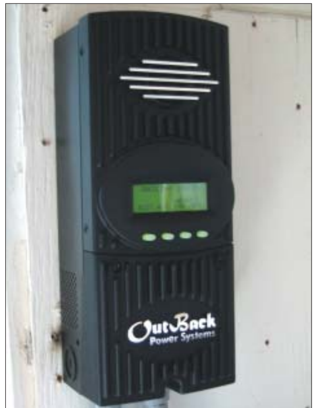
Photo 8. 60 A max power tracking PV charge controller
