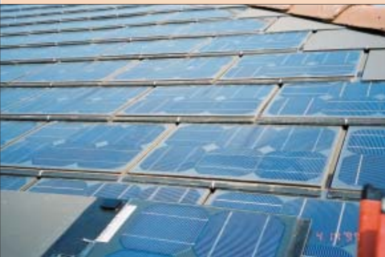
Photo 2. PV modules as roofing material
