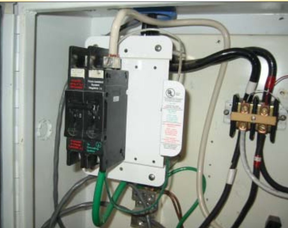
Photo 12. Stand-alone PV ground-fault protection device
