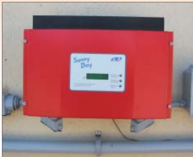
Photo 10. Utility-interactive 2.5 kW inverter
