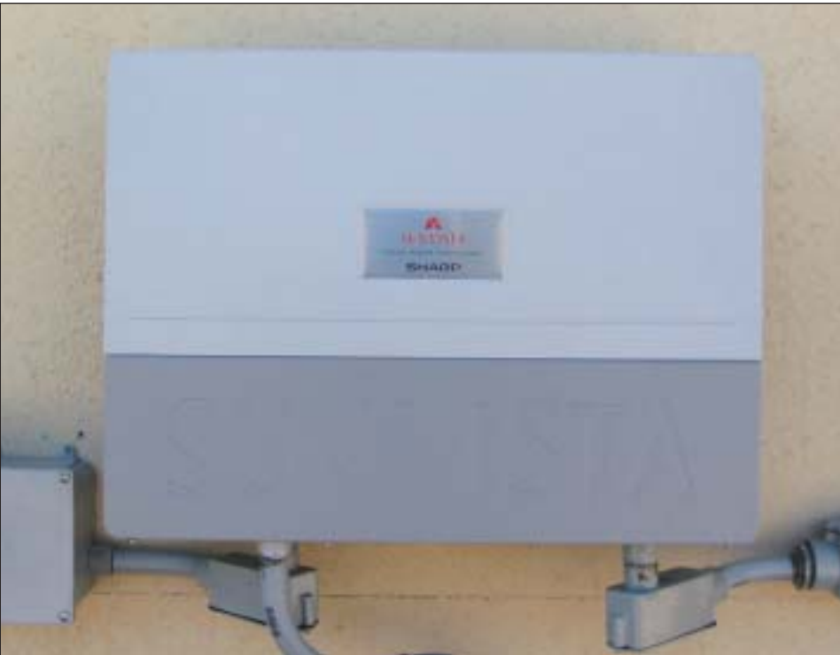
Photo 11. Utility-interactive 3.5 kW inverter
