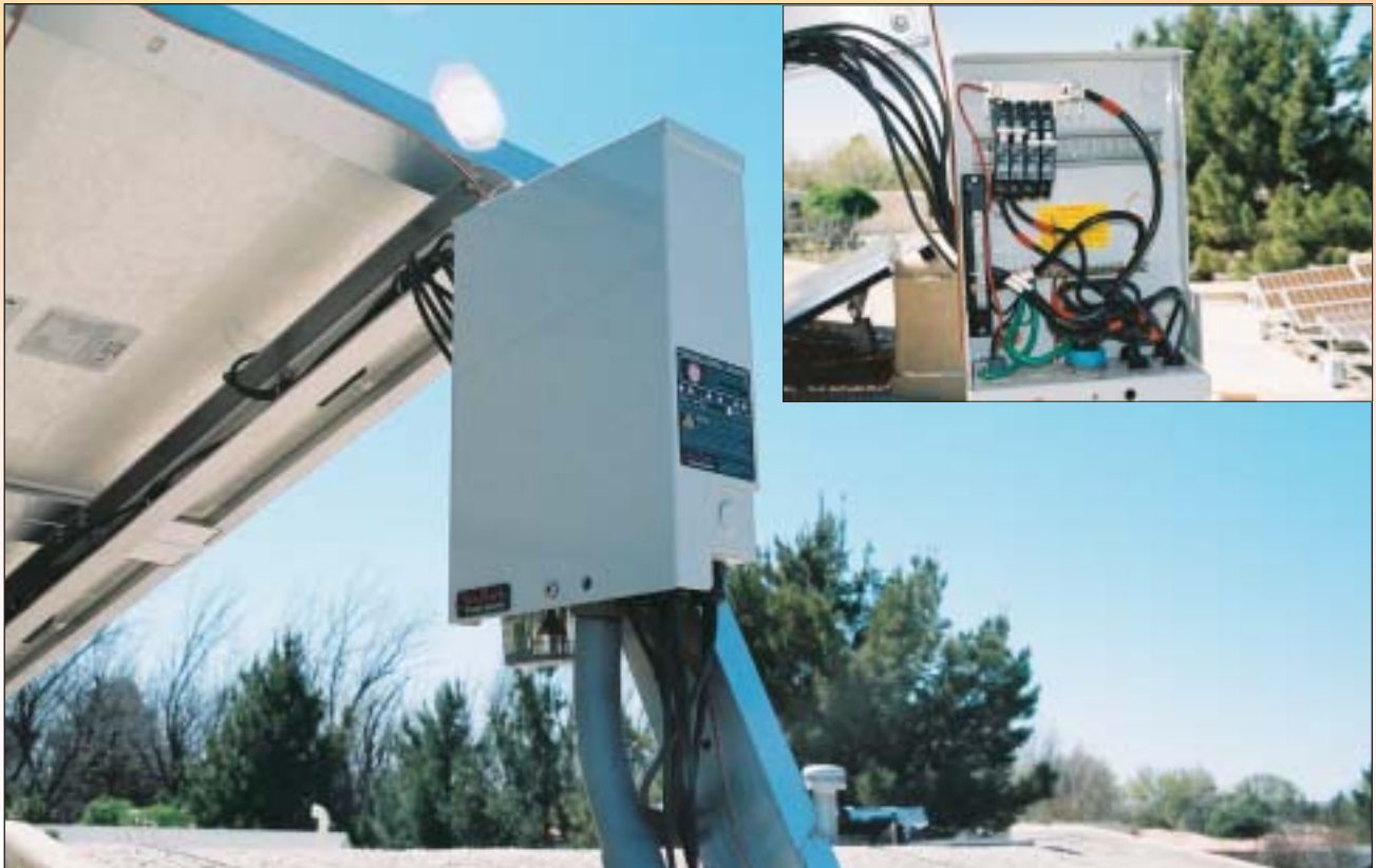
Photos 5 and 5A. PV combiner with circuit breakers
