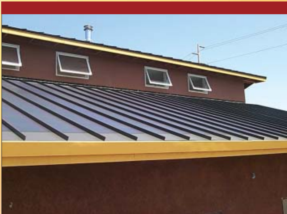
Photo 3. PV modules laminated to metal roof
