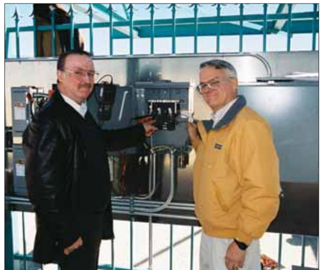
Figure 5. The author, right, and Albuquerque, NM, Electrical Inspection Supervisor Hal Kissinger inspecting a load-side connection
