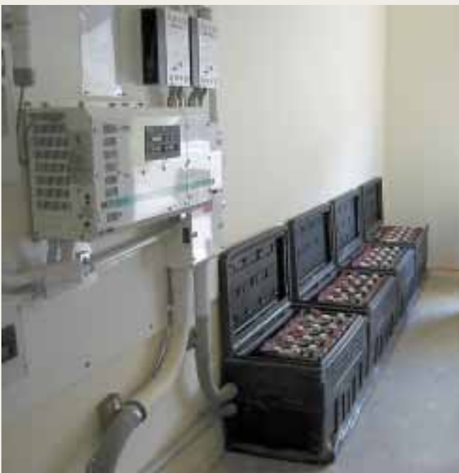
Battery row—sixteen L16HCs in four polyethylene tool boxes.
