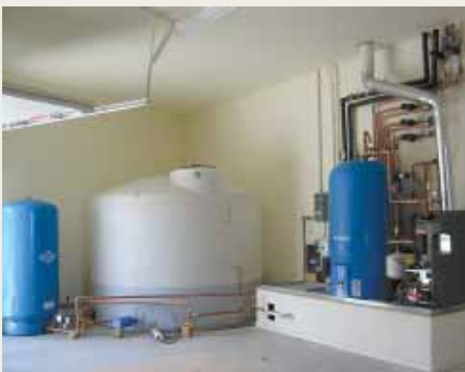
The potable water and radiant floor system components live in the garage.
