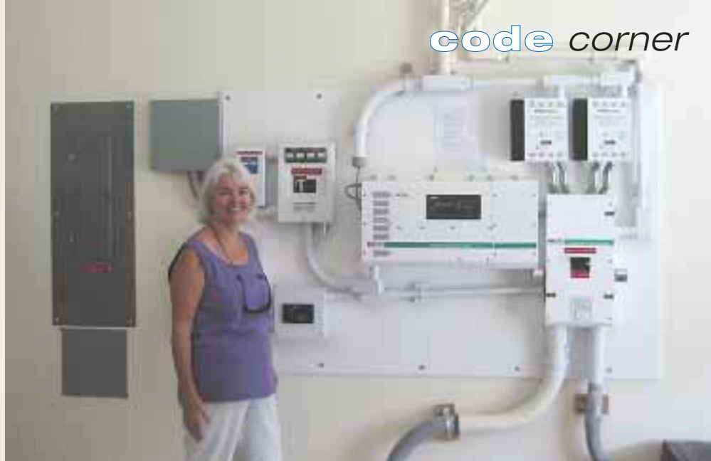
Judy LaPointe in front of the PV power panel.
